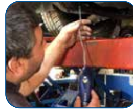
Leak from the compressor shaft.
